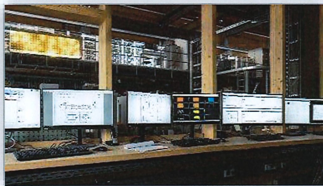
Smart Energy System Simulation & Control Center
